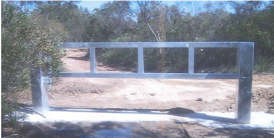
Figure 3: Gosford City Council Custom Designed Gate
